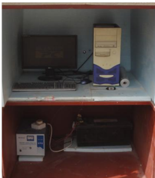
Fig (6) Computer, inverter, System battery charging
